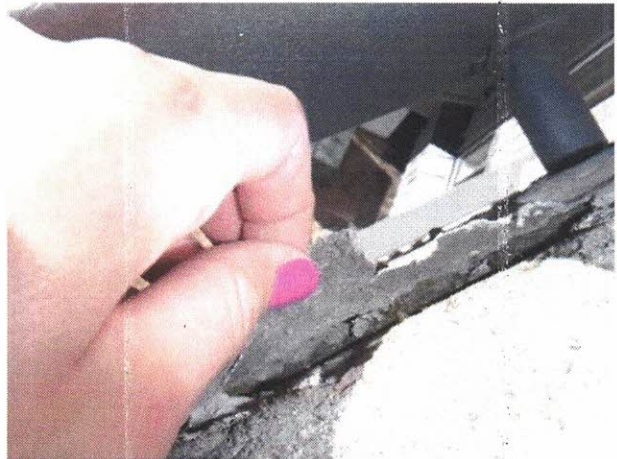
Photo 13: Deteriorated joint sealant at edge of balcony.
