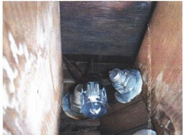
Photo 23: Awl was able to penetrate through the plywood sheathing with little force. (Unit 304)
