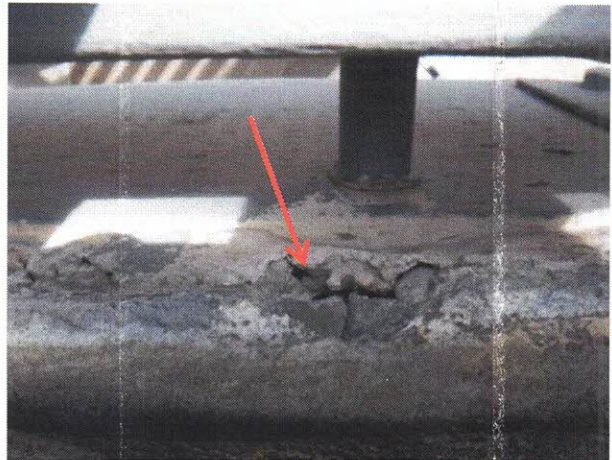
Photo 11: Guardrail is attached through face of rim joists. Note void in concrete at edge of balcony.
