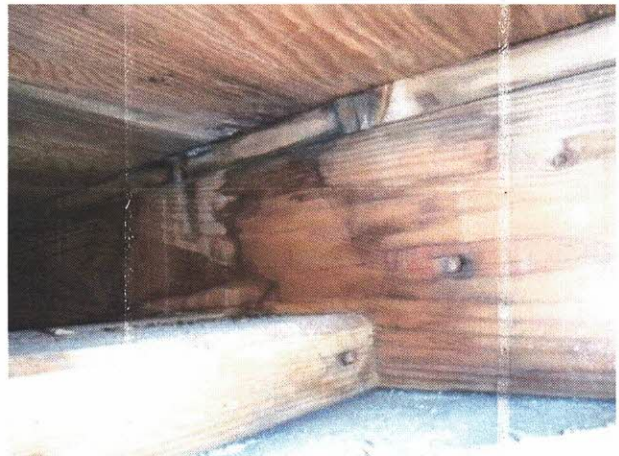
Photo 27: Staining is apparent on sheathing and joists. (Unit 302)
