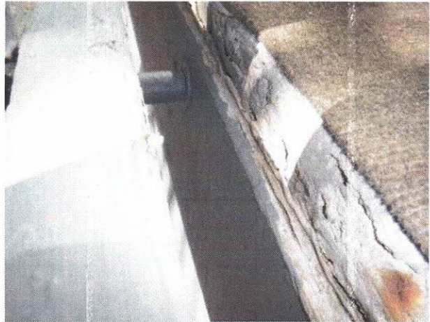
Photo 15: Deteriorated joint sealant at edge of balcony.
