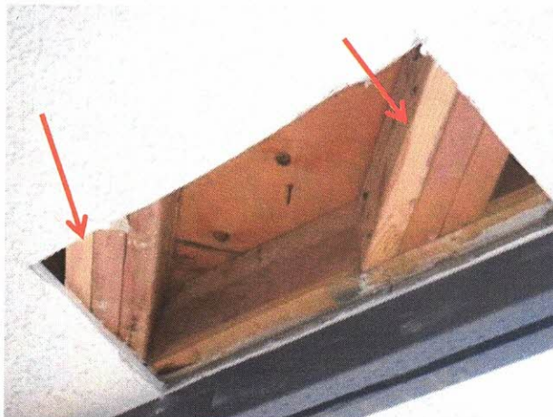
Photo 34: Exploratory opening at soffit. Note sistered joists (arrows). (Unit 104)
