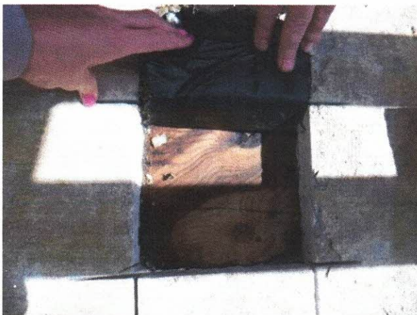
Photo 18: Exploratory opening into concrete topping slab. Note the presence of a black membrane over the plywood sheathing and staining on the sheathing. (Unit 404)
