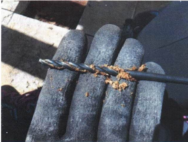
Photo 20: Plywood shavings are moist and soft. (Unit 404)
