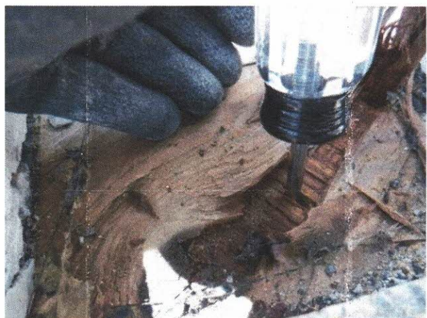
Photo 19: Awl was able to penetrate through the plywood sheathing with little force. (Unit 404)
