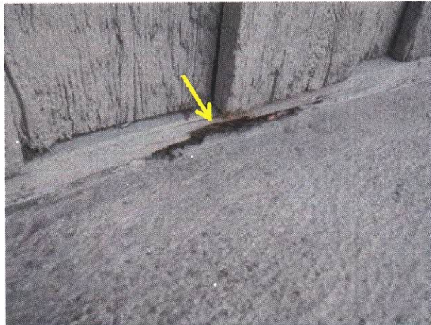
Photo 8: Deterioration of wood trim adjacent to balcony. Note the balcony at this location has been coated.
