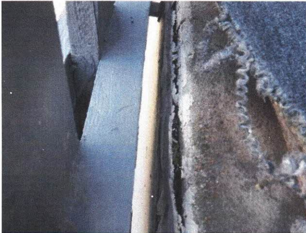
Photo 12: Deteriorated joint sealant at edge of balcony.
