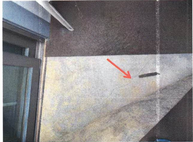
Photo 3: Crack in concrete topping slab below carpet covering. Note yellow residue from failed adhesive.
