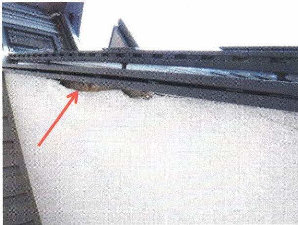
Photo 16: Popcorn finish at soffit is deteriorated.
