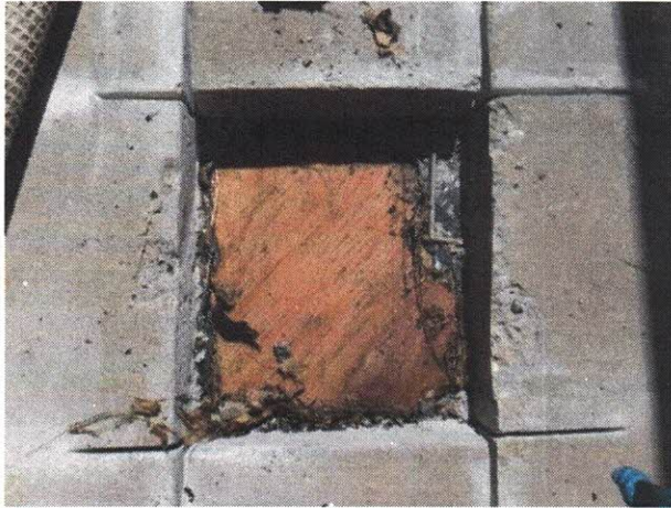
Photo 24: Exploratory opening into concrete topping slab. Note lower right-hand corner of sheathing is stained. (Unit 407)
