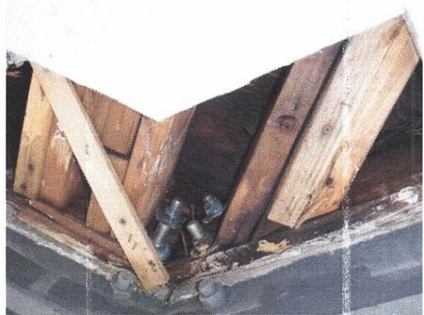
Photo 21: Exploratory opening into soffit. (Unit 304)
