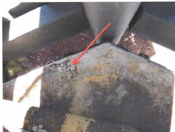
Photo 4: Concrete deterioration at edge of concrete topping slab.
