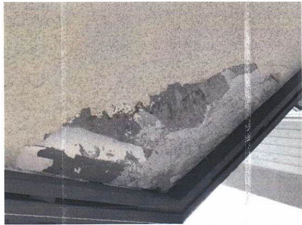
Photo 17: Popcorn finish at soffit is deteriorated.
