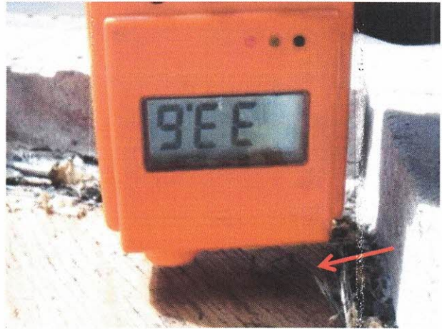
Photo 25: Moisture content reading of 33.6 percent at plywood sheathing. (Unit 407)
