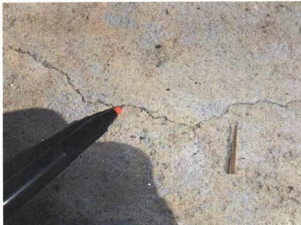
Photo 2: Crack in concrete topping slab.
