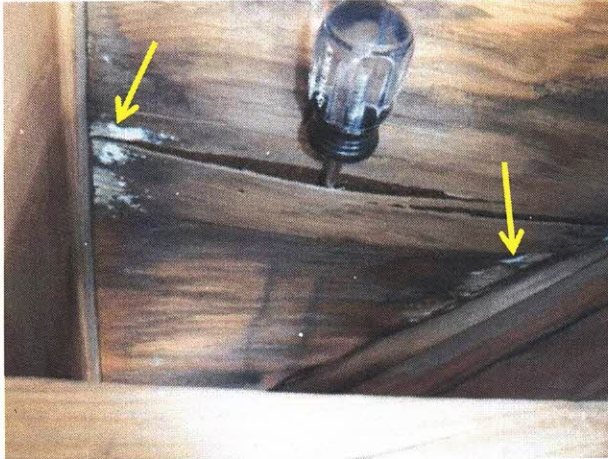
Photo 28: Organic growth is present on the plywood sheathing (arrows) and the outer layer of the sheathing is no longer bonded. (Unit 302)
