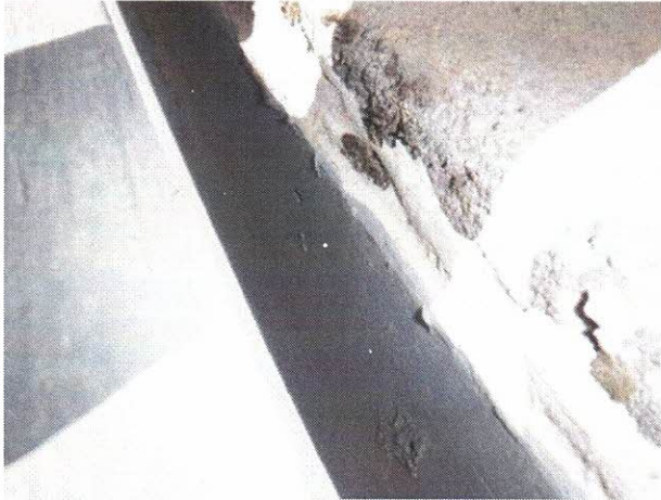
Photo 14: Deteriorated joint sealant at edge of balcony.
